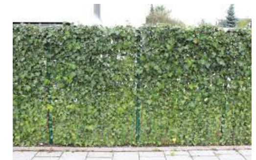
TRANSFORMER FENCE WITH IVY
